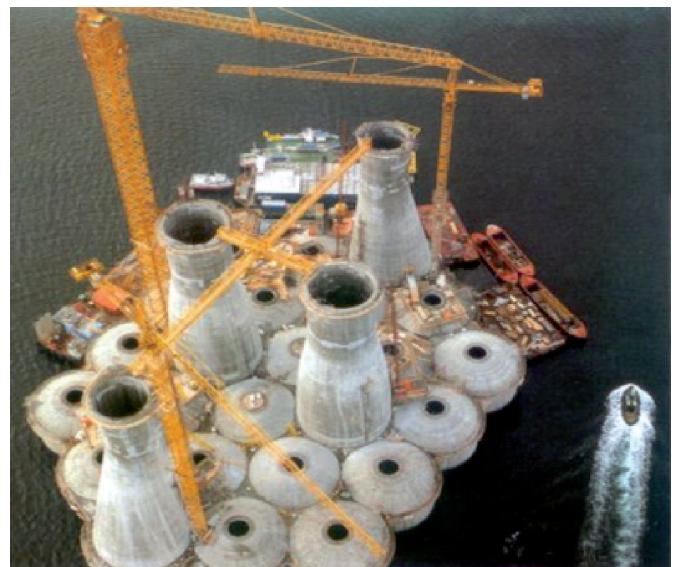
(a) The Sleipner Platform prior to collapse
